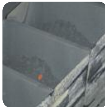
Hot clinker conveyor
